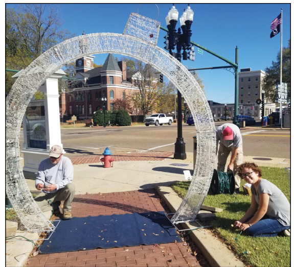
It was a warm day when Joel Crosno, Clayton Lee, and Alexandria Hassell worked to erect the beautiful holiday decorations on the Downtown Plaza.
